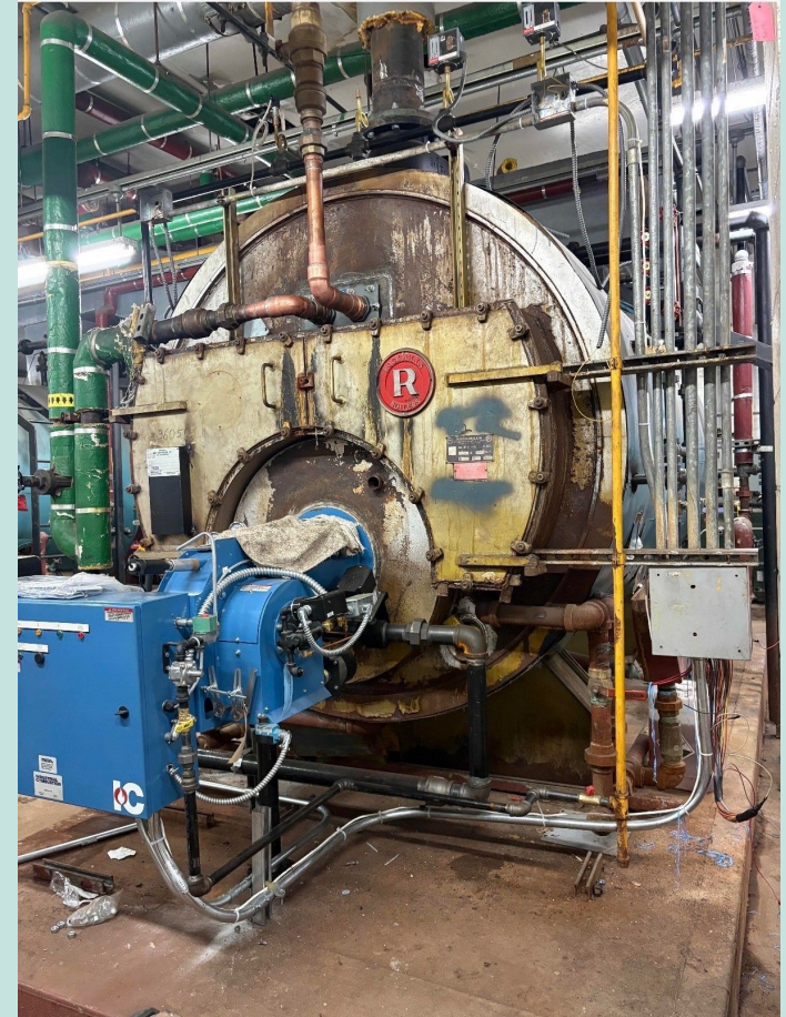
SGL boiler after renovations.
